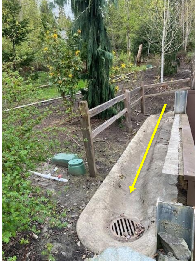
Runoff sheet flows east toward the adjacent Aegis Living property and is collected by an interceptor trench along the property line.
